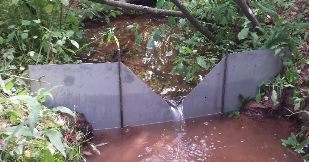
V-notch weir to measure water flow.
