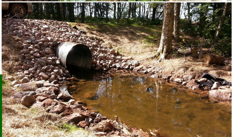
Photos (from top to bottom): Before, during, and after culvert replacement at Black River. The downstream end of the culvert is no longer "hung" which required fish to jump up into the culvert, now fish can easily swim through this larger culvert. Farm equipment can also more easily use this improved crossing, and not worry about a small culvert washing out during a big storm.
